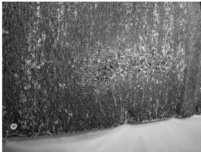
Fig. 13: Condition of the perforated Whisper® NBO-40-A3 absorber element after 30 theoretical years; details of the scorched surface
